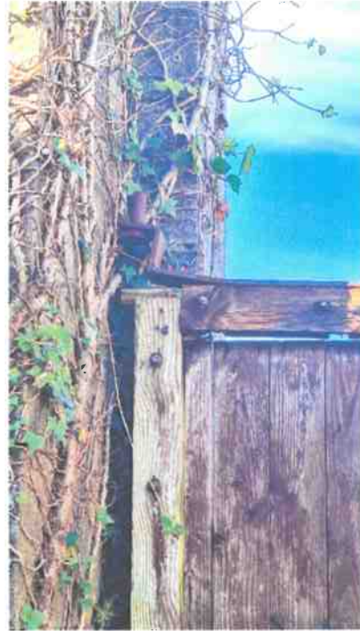
Fig. 46 South pier was listing to the north
