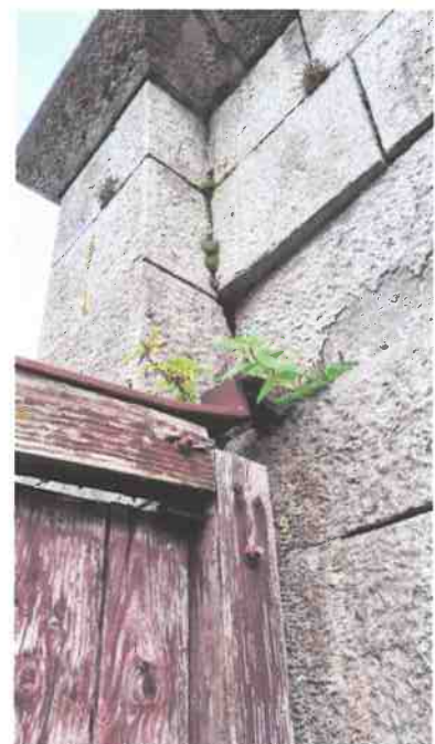
Fig. 7 top hinge pulling away from pier
