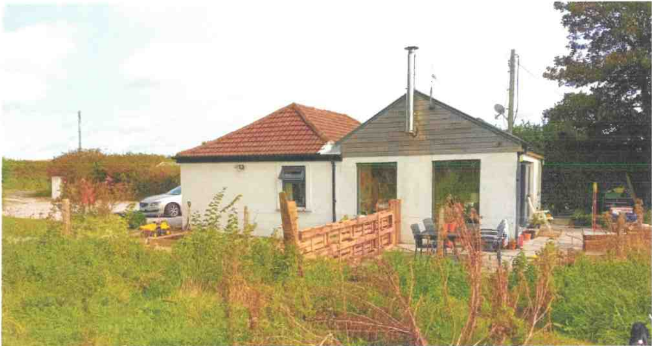
View from South-West. Pre-existing Gable on the left, Extension on the right
