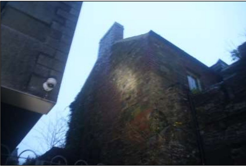
Plate 4 Existing main courthouse (rear) which is not illuminated – cracks in stonework a potential roost feature.
