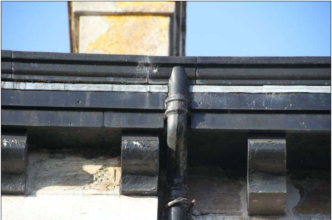
• Fig 29. Gutter detail to Courthouse and flashing and possible steel channel detail to be investigated.
