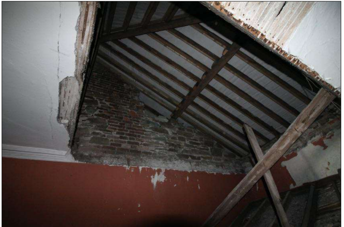
• Fig 105. Room. 20 Collapsed ceiling.
