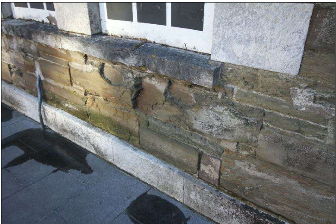
• Fig 28. Eroded pointing and severe erosion in face bedded stones.
