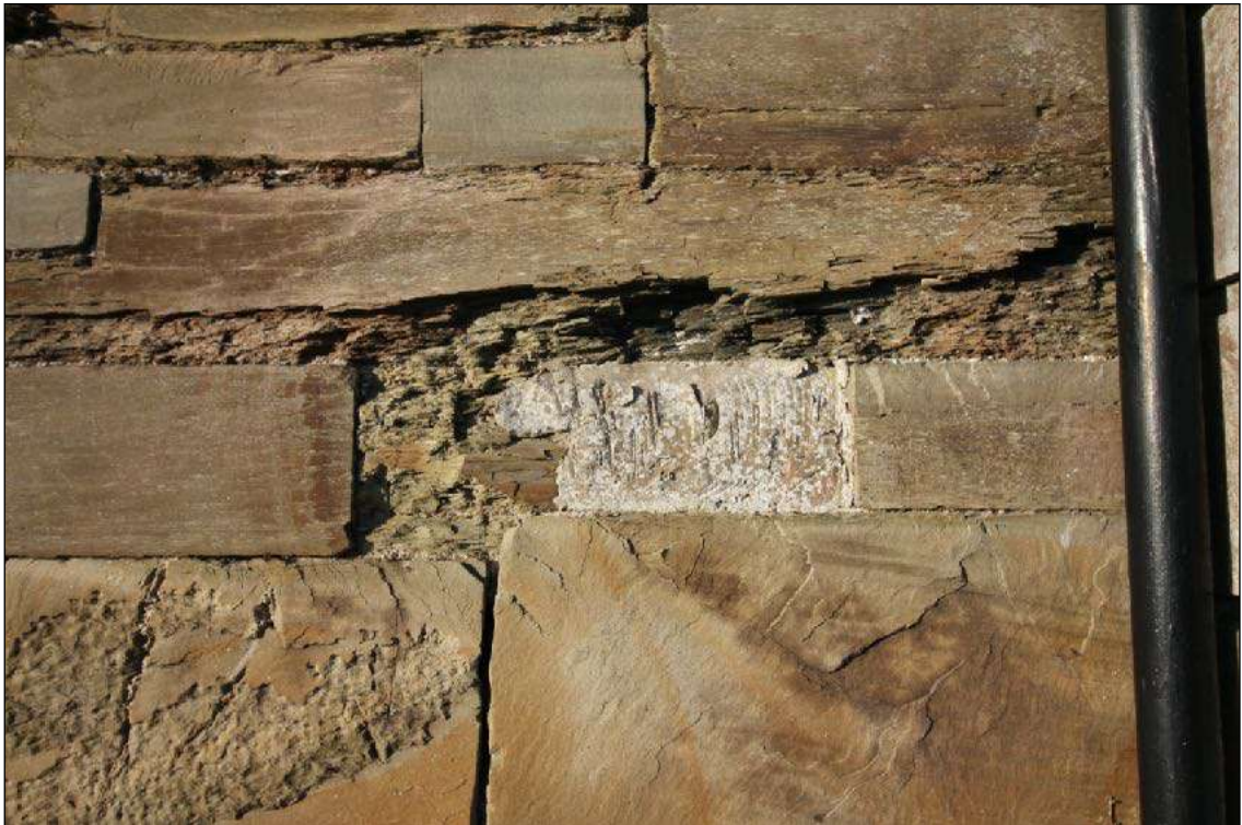
• Fig 27. Eroded pointing and severe erosion in face bedded stones.
