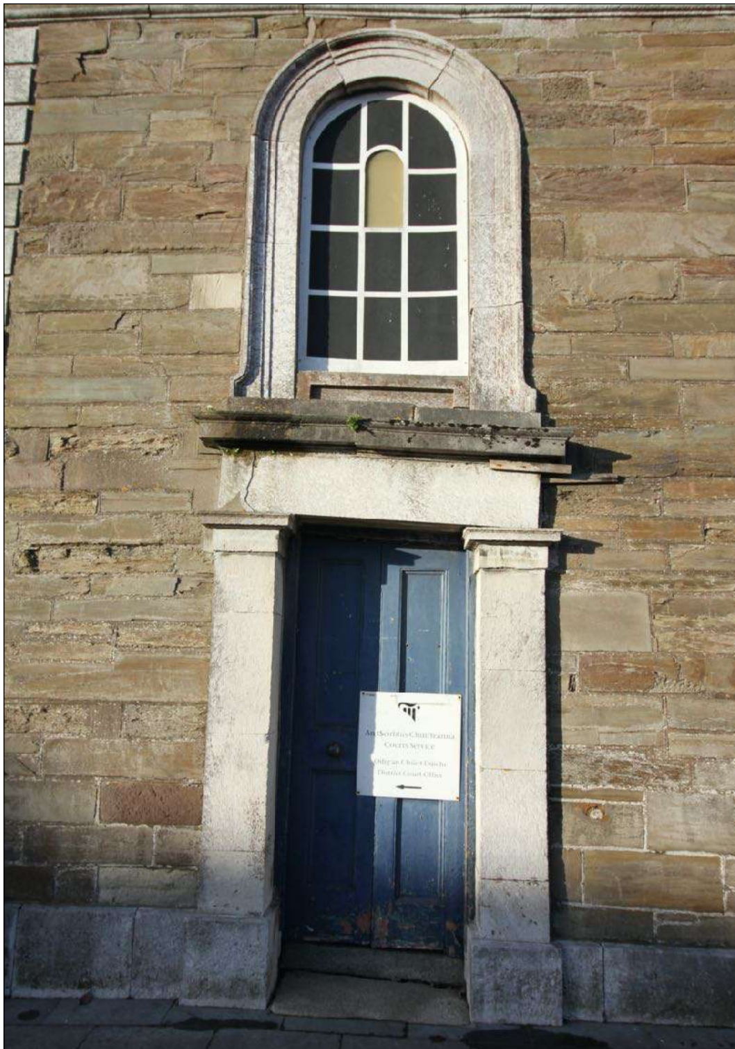
• Fig 31. Settlement in South East corner.
