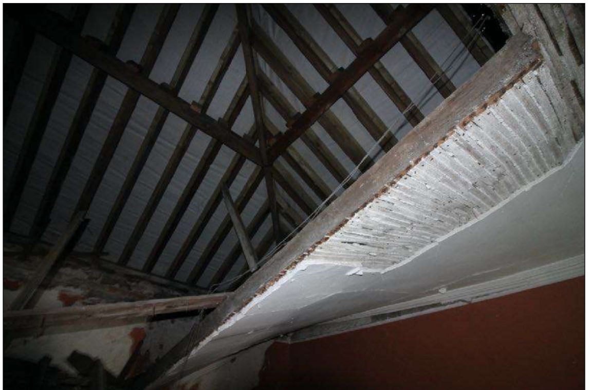
• Fig 106. Room. 20 Collapsed ceiling.
