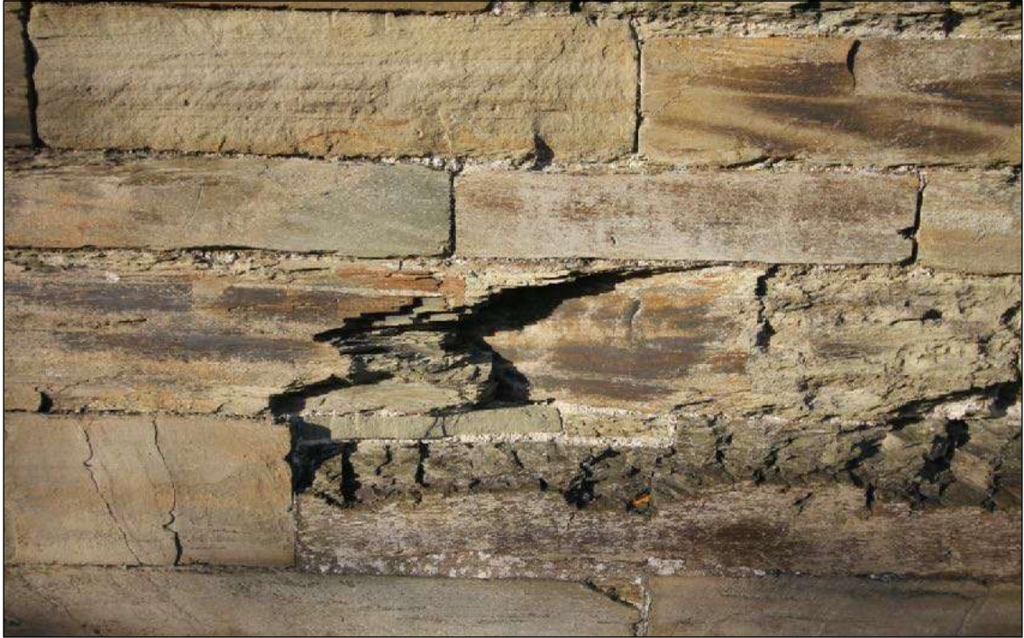
• Fig 25. Eroded pointing and severe erosion in face bedded stones.
