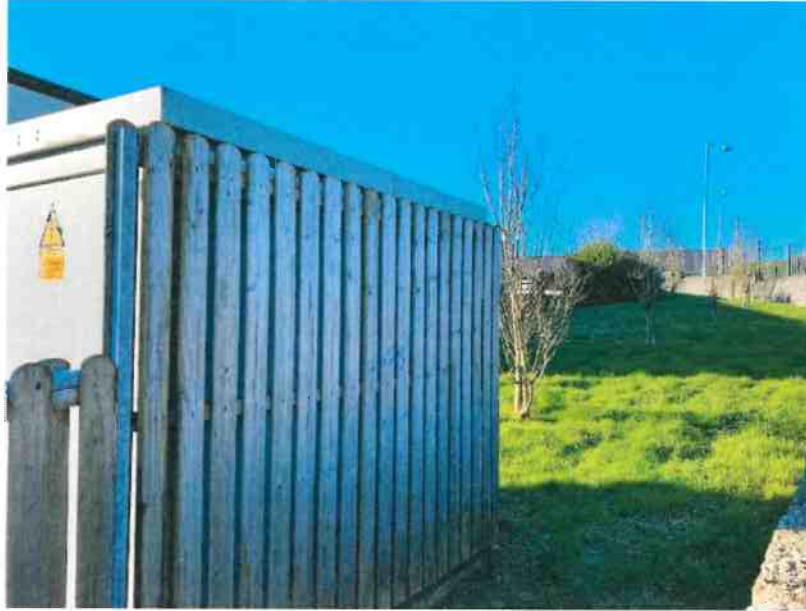
Existing ESB Substation on site which has been partially cladded in timber.
