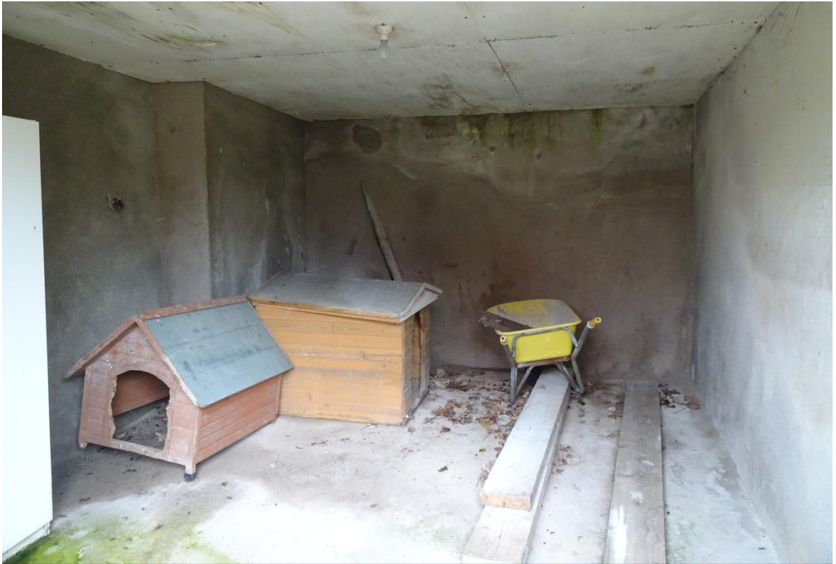
Plate 8 Interior of storage shed in northwest corner of site. Rear wall is part of demesne wall.
