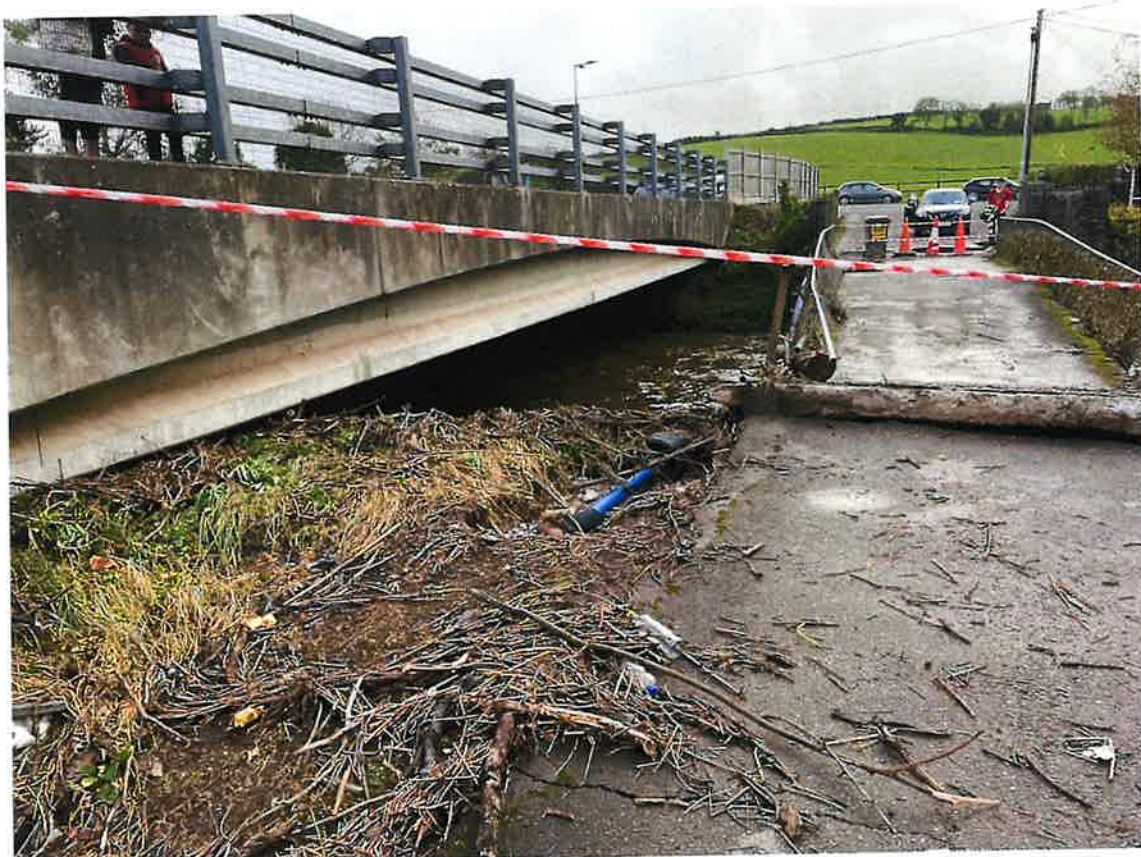
Figure 4: View from west over damaged Broomfield Ridge Bridge with Tir Cluain bridge to left of picture
