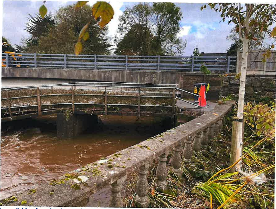
Figure 3: View from South East of damaged bridge (November 2023) with Tir Cluain Bridge in background
