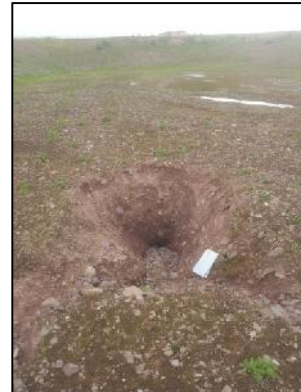
Photo 4 Swallow Hole KF14 at base of attenuation pond at IDA site in Ballyadam
