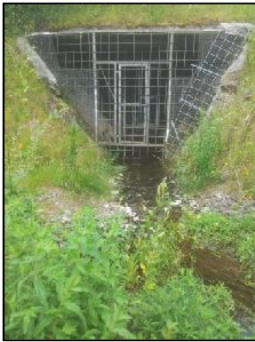
Photo 3 Swallow Hole KF15 at Cúl Ard Housing Estate, Terrysland
