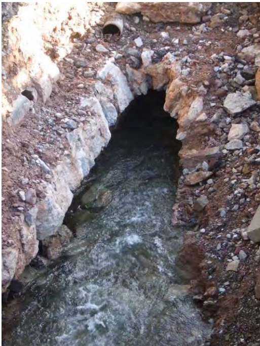
Old stone arch culvert (collapsed during flooding in Aug 2012)
