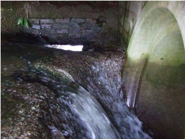
Inlet to Cascade and Overflow Pipe to IDA Siphon
