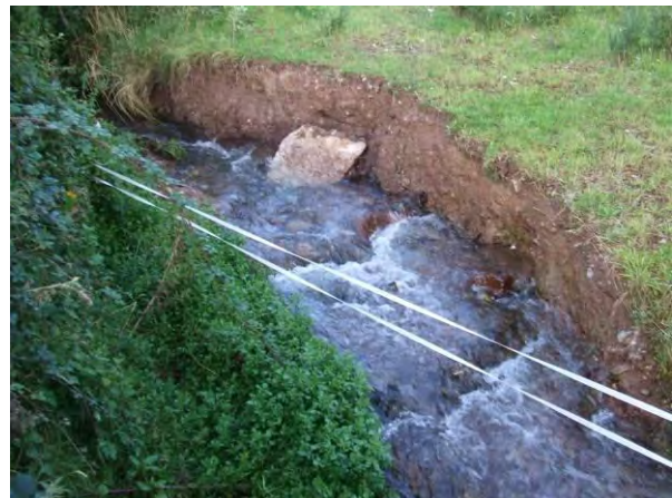
Erosion on left bank upstream
