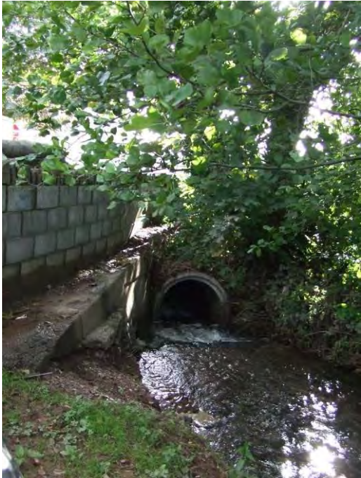
Circular pipe inlet
