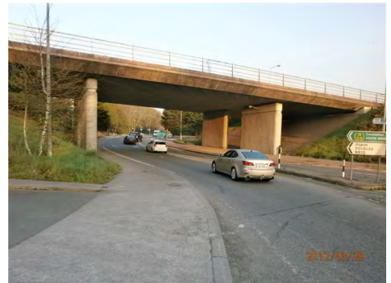
Picture 2: Standing at Roundabout facing west towards right turn for slip lane onto N28
