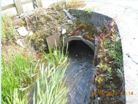
Poor culvert inlet
