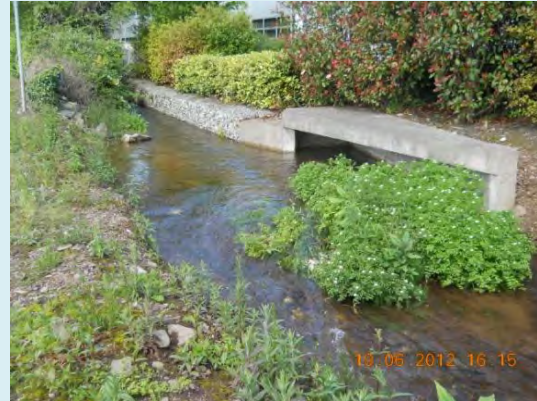
Localised sediment at outfall
