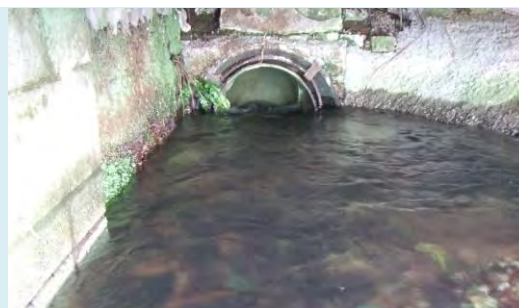
Irish Rail Siphon
