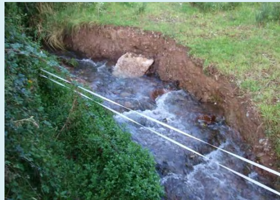
Evidence of erosion upstream
