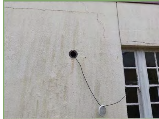
Plate 3.2.4 View of extraction fan out-pipe associated with the ground floor kitchen.
