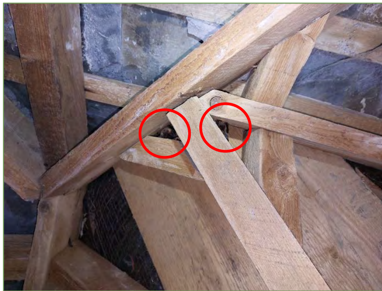
Plate 3.2.7 Two Brown Long-eared Bats (red circles) located within the joinery apex of the western attic section of the former Garda Station
