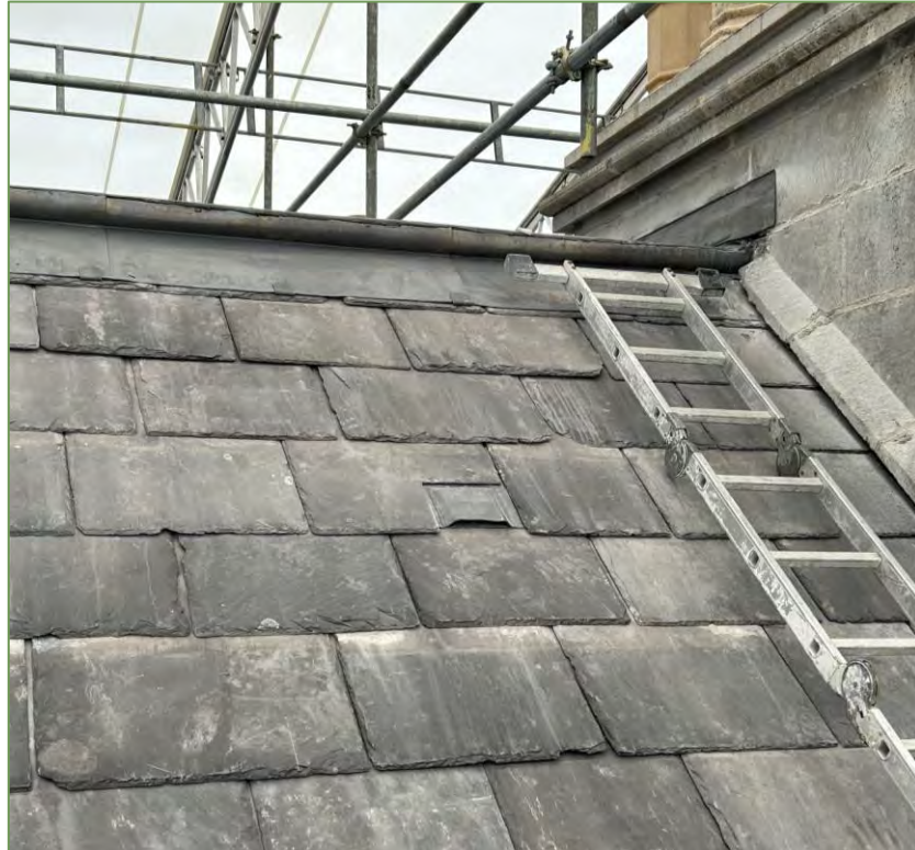
Plate 5.2 - Example of a lead bat access tile.
