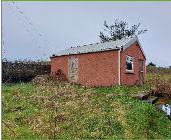
A3. Outbuilding associated with the existing building located to the south, photographed from the east facing southwest.
