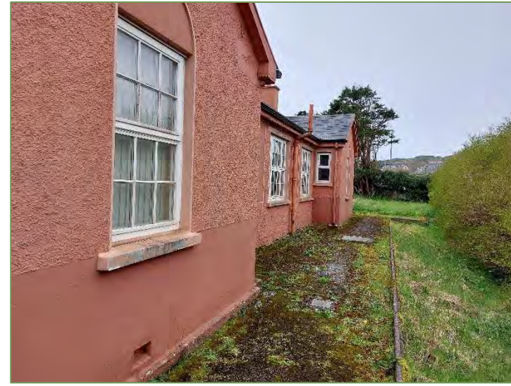
A2. View of the north-facing façade of the existing building facing west.
