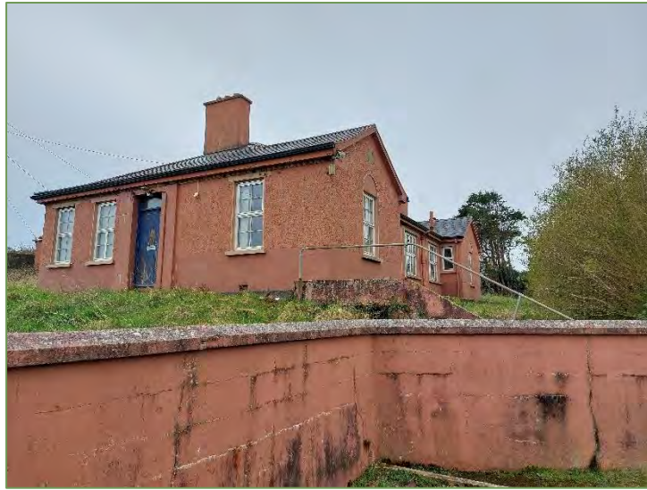
A1. View of the northeast corner of the existing building at the proposed site, previously occupied as Goleen Garda Station, photographed from the L4401.
