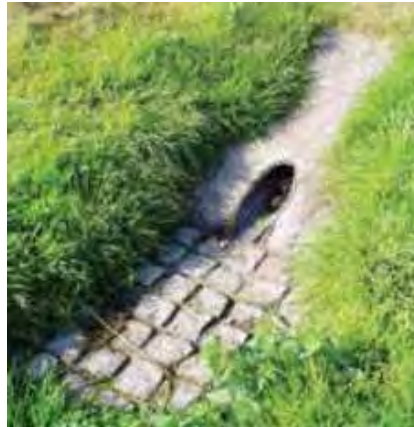
Figure 8: Basin inlet/outlet with concrete surround and cobbled spillway to prevent overgrowth & erosion
