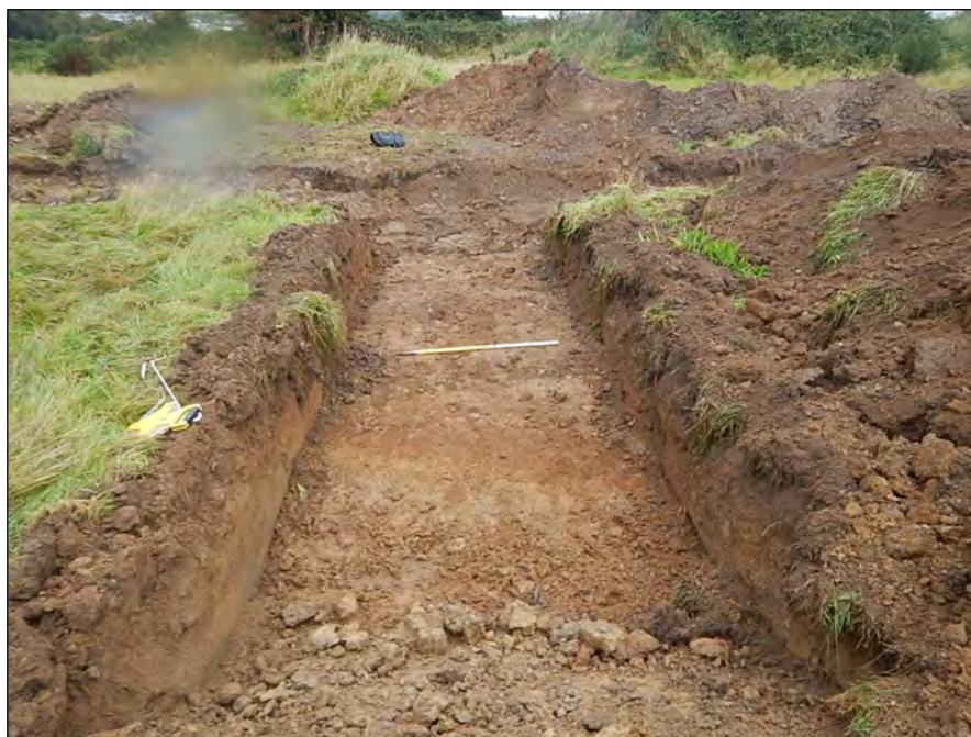
Plate 26: Trench 18, showing southern edge of F13 visible in trench extension, looking north
