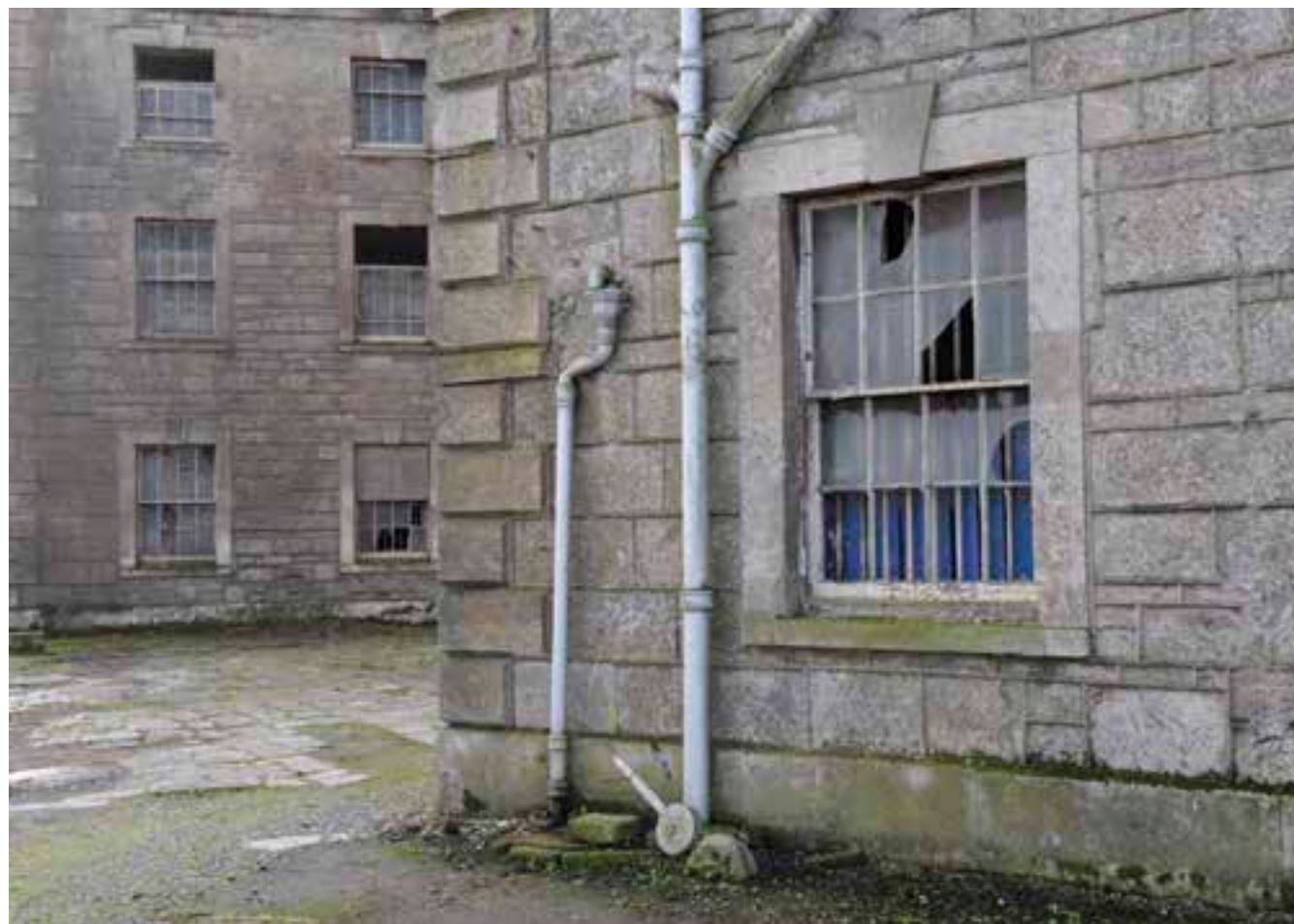
Fig. 3.85 The historic Store Houses are fine examples of limestone and granite industrial buildings, that are unfortunately in serious decay.
