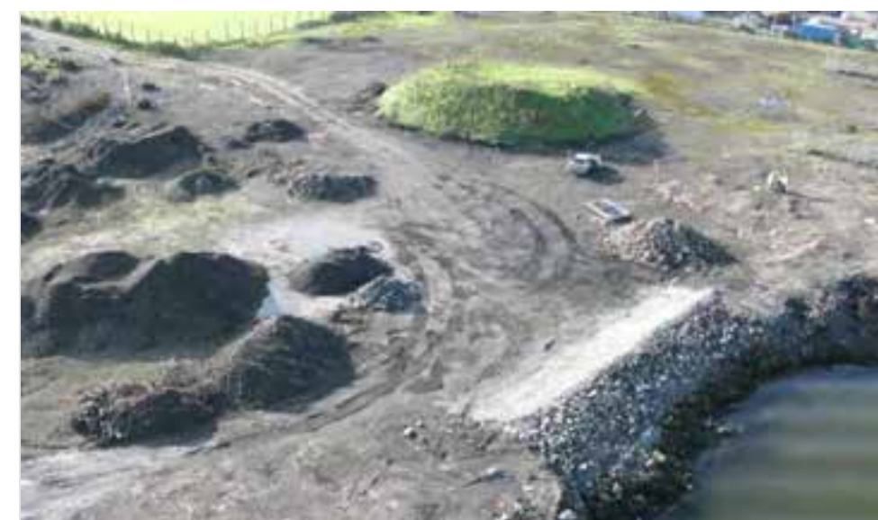
Fig. 3.51 East Tip prior to remediation.
