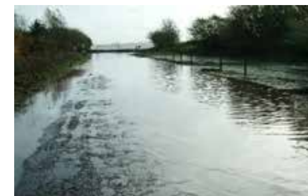
Fig. 3.12 Flooding on the road approaching Haulbowline.
