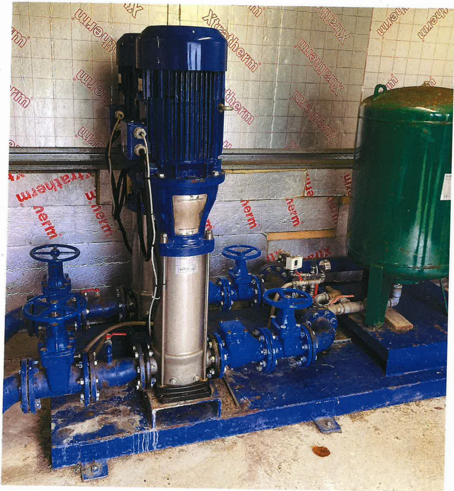
Inside Pump House View
