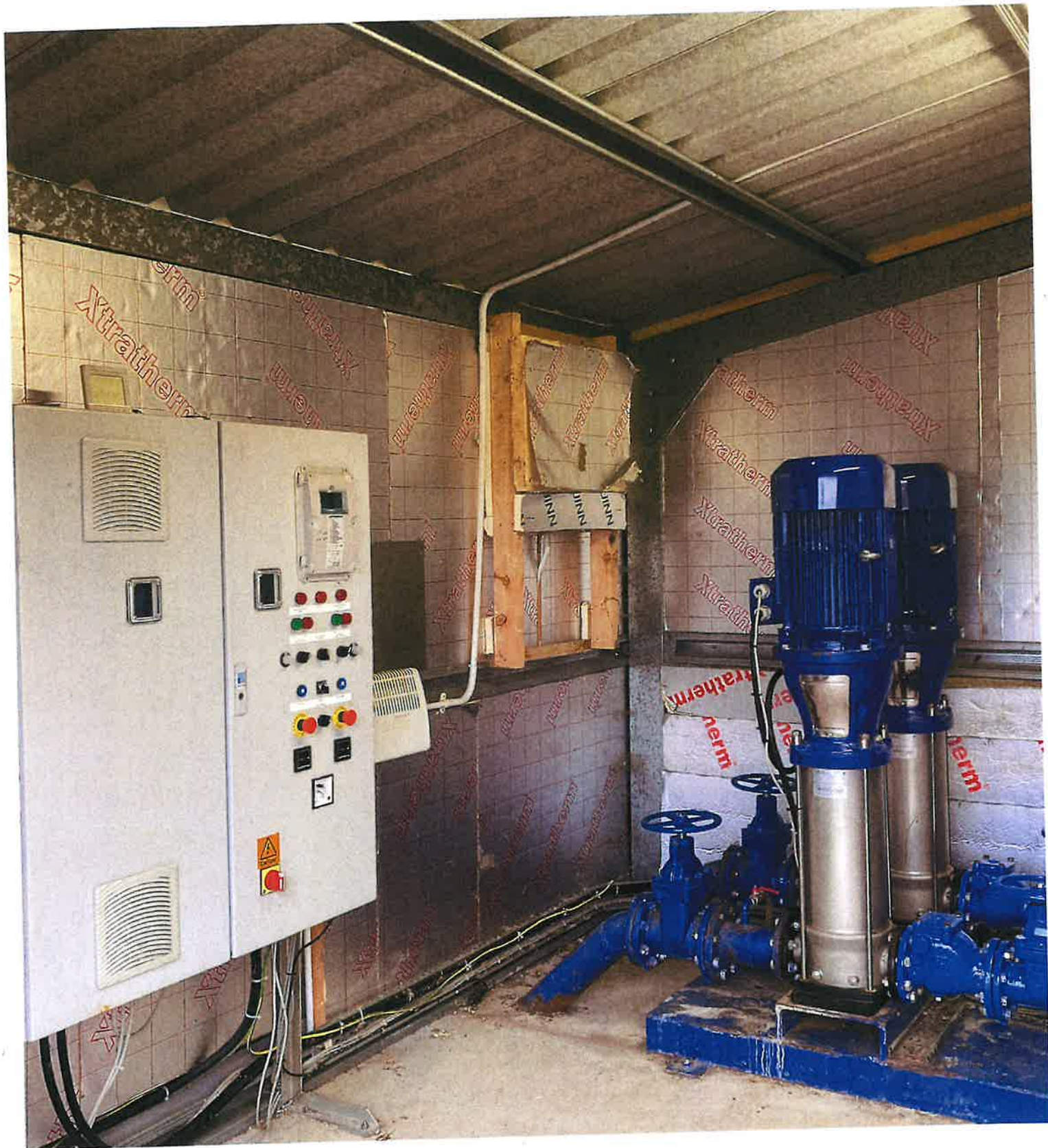
INSIDE PUMP HOUSE VIEW
