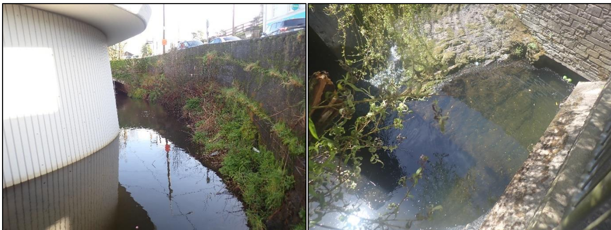
Plate 3: View upriver from weir (left), view of pond below weir (right). Entrance to culvert can be seen in right background.
