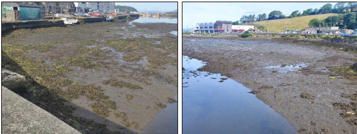
Plate 4: View of south (left) and north (right) views of the marina from over the culvert exit.
