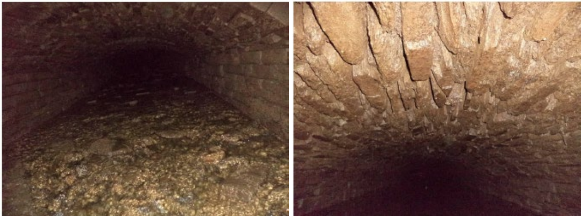
Plate 1: Image of interior of culvert (MWP, 2018). Plate 2: Image of interior of culvert (MWP, 2018).
