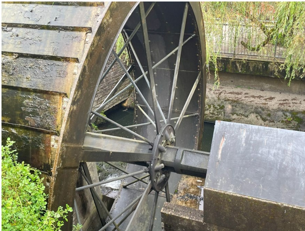
Plate 4: View of culvert inlet behind replica mill wheel on site of former mill.
