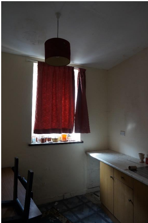
66 Interior of Building C. Walls have been dry- lined. Not original to build.
