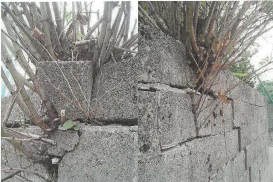
Photograph 1.4 Japanese Knotweed breaking through cavity blocks resulting in a structural crack in the wall of a garden in Co. Cork (Source: Lisa M. J. Dolan, Ecosystem Services)
