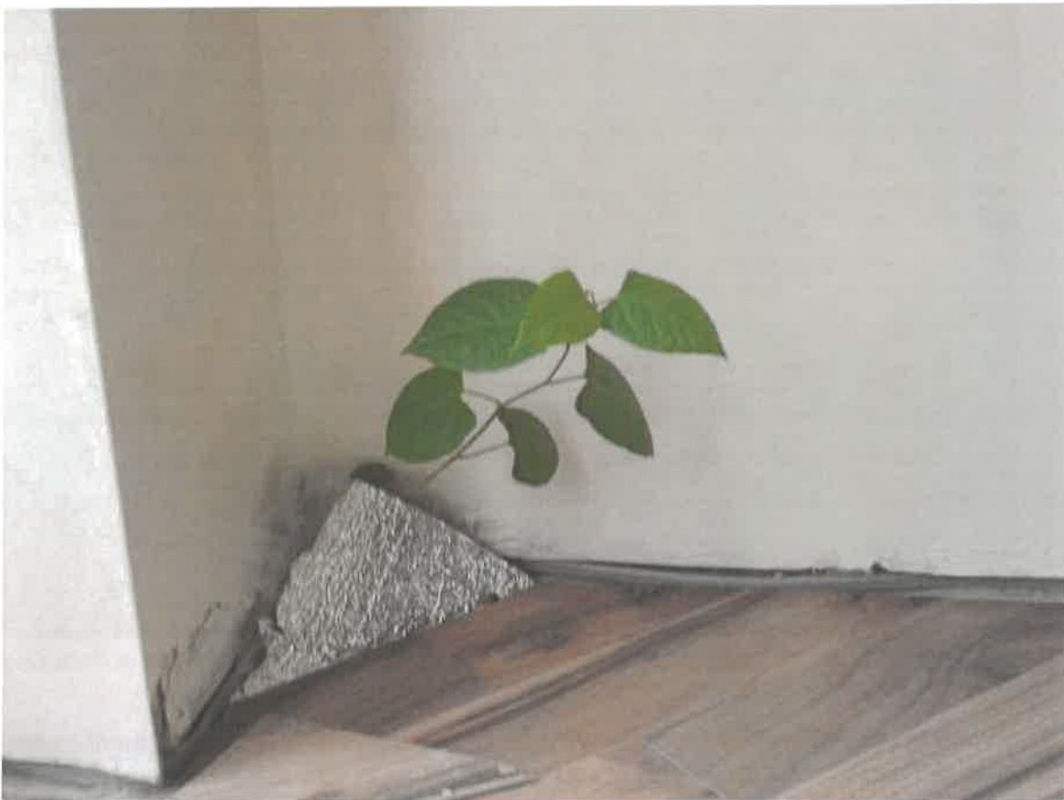
Photograph 1.2 Japanese Knotweed having broken through a weakness in the structure and gained internal access to a private dwelling in Co. Cork
