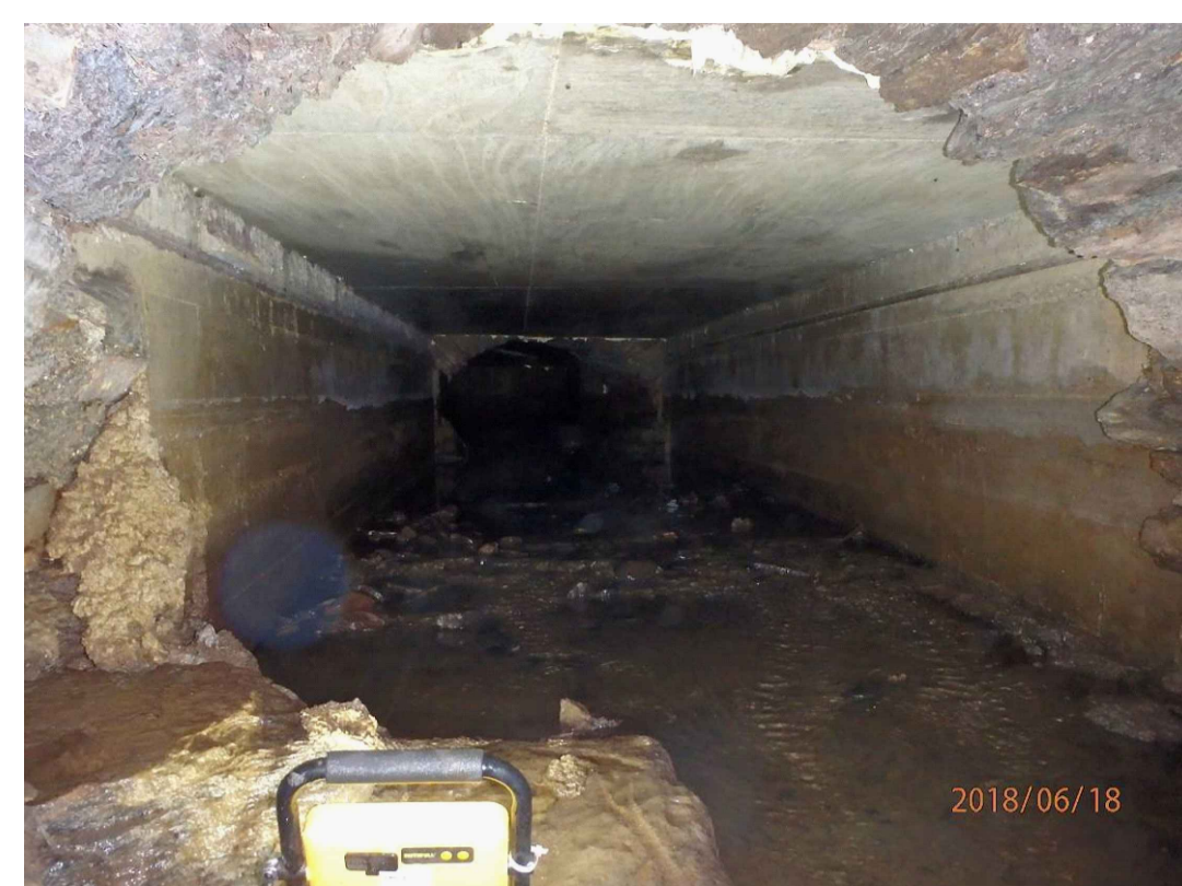
VIEW 1 - TAKEN LOOKING UPSTREAM INTO ALLEY STREAM BOX CULVERT (WITH MASONRY ARCH AT BUILDING LINE TO FRONT)
