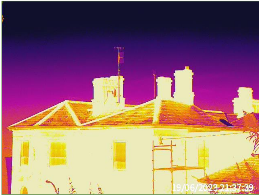
A9. Thermal image from a limited survey of Rockenham House on 19 th July 2023.
