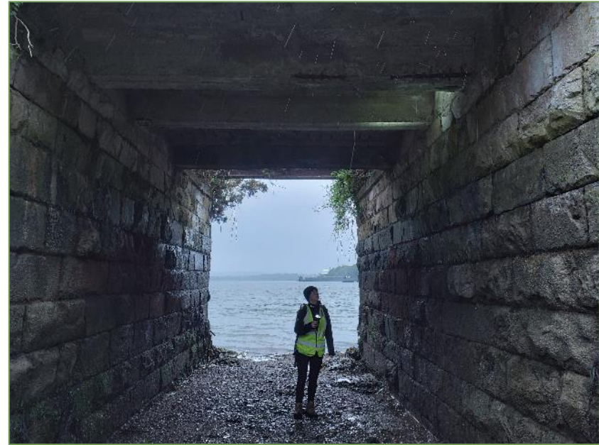
A4. Showing artificial bridge deck (No. 4) and parapet to be replaced with a 300mm wide bridge deck and railing. This deck and parapet were inspected at low tide to aid accessibility for surveyors. Minor crevices were recorded that have low potential as roosting features for crevice-dwelling bats.
