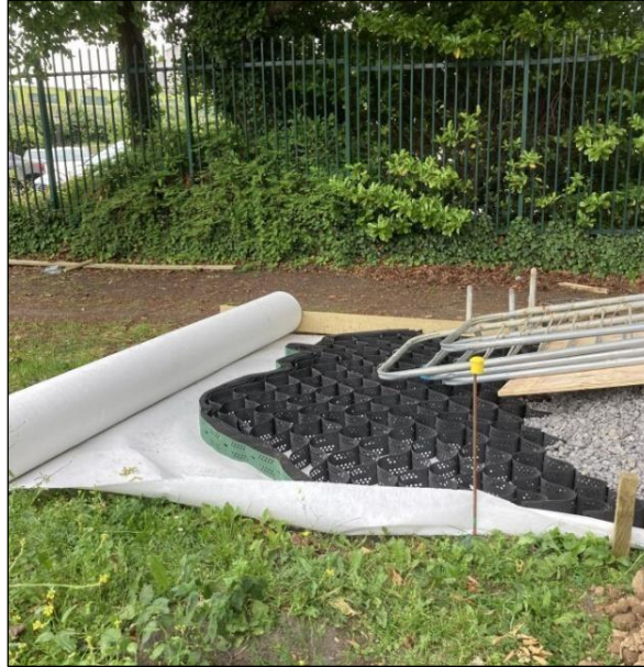
Plate 1-3 - Fill cellular material confinement system to evenly distribute loads across the proposed pedestrian and cycle path.
