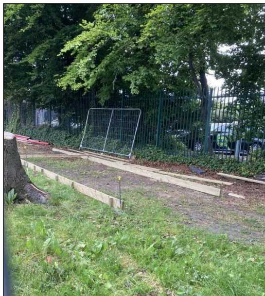
Plate 1-2 - Prepare the proposed pedestrian and cycle path for the cellular confinement system.
