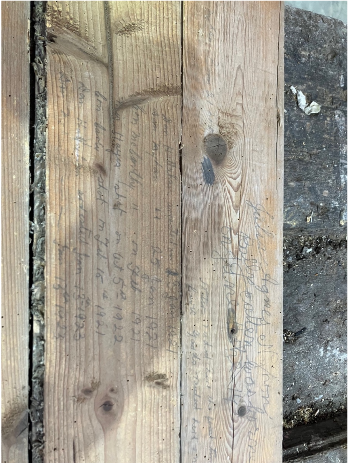
This is an interesting multi-phase building that would benefit from further recording and research.
