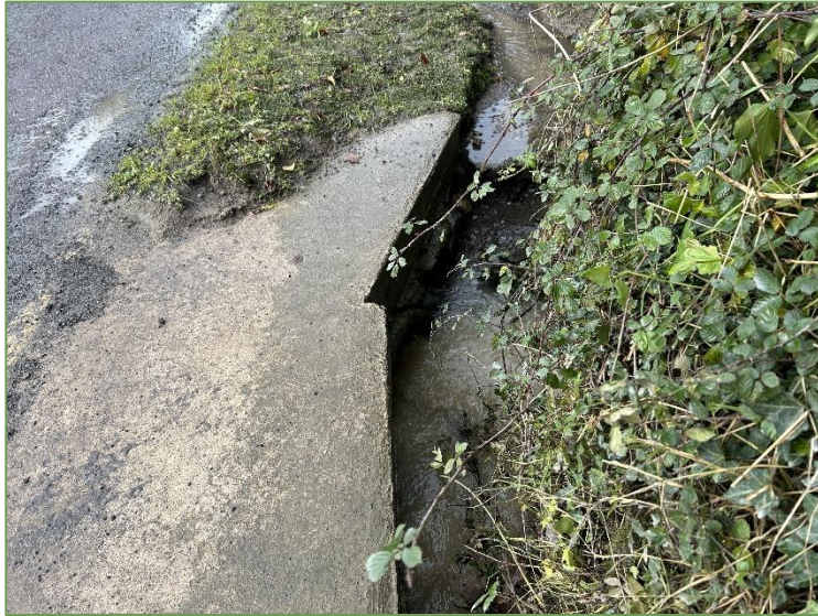
A3. Culvert carrying the Knocknabohilly Stream underneath the Bandon Road (L3234) at the north of the scheme.
