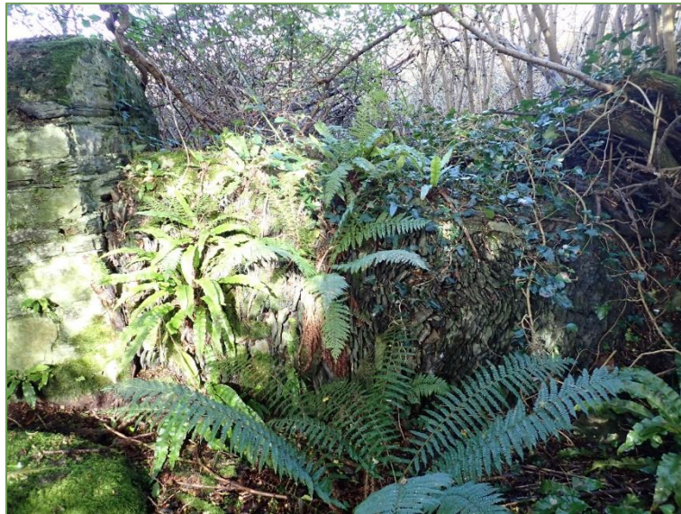
Plate 3.2.9 – Stone wall (BL1) present within woodland at the southern extent of the site.
