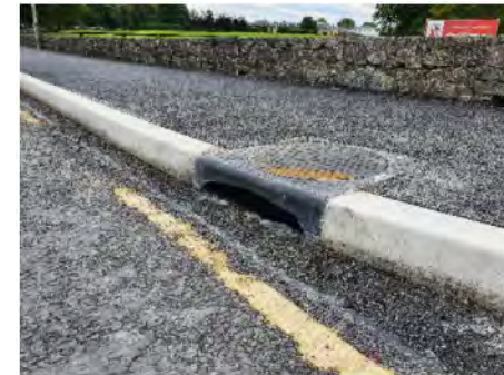
SIDE ENTRY GULLY
