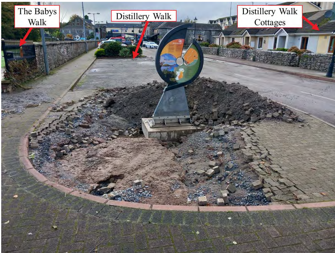
Figure 75: Scour Damage at Distillery Walk
