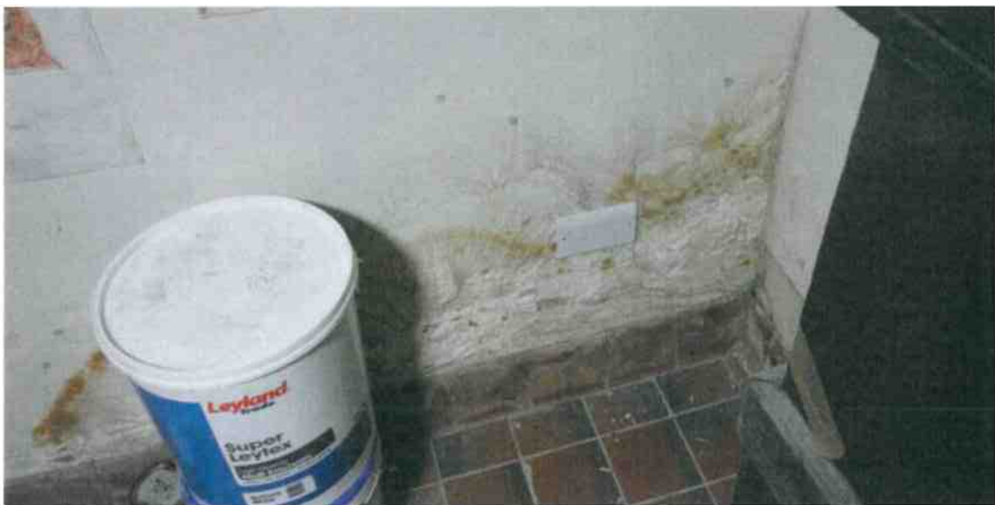
• Fig 79 & 80. Rot indications in rear rooms to GF Eastern block.
