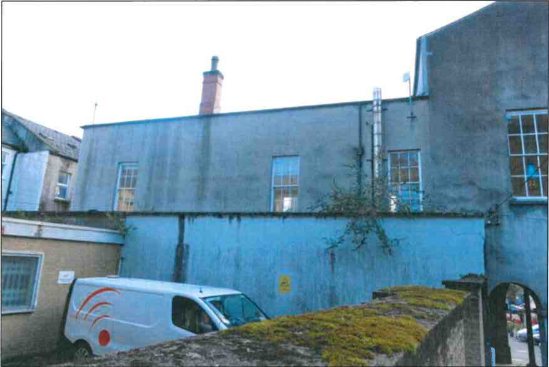
• Fig 19. North elevation, East end and EIR car parking area. Flat roofed structure behind main building.
