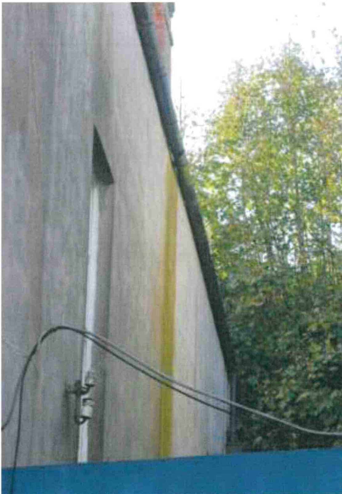
• Fig. 83. Leaking rear gutters.
