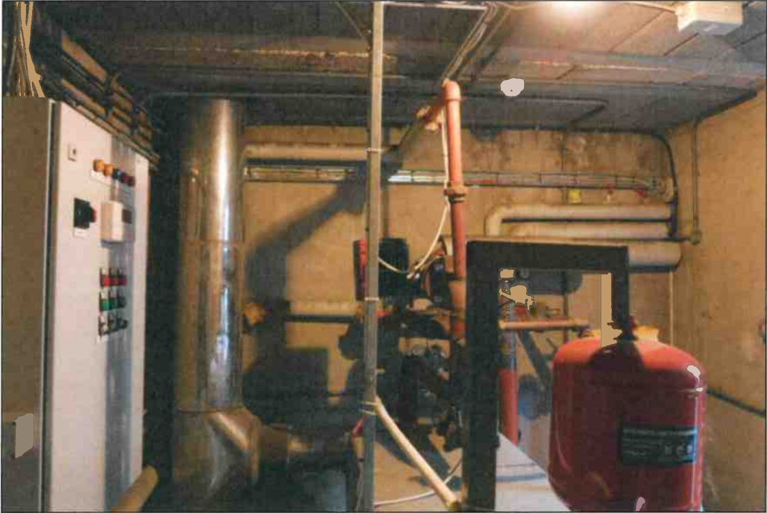
• Fig 73. Boiler room No. 13.
