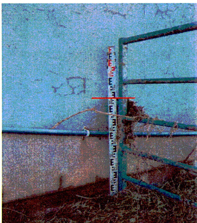
Photo 4 Trash level on gate at pump house beside Baile Mhic Íre Bridge
