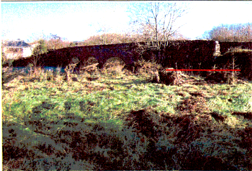
Photo 3 Trash level on vegetation upstream of Baile Mhic Íre Bridge
