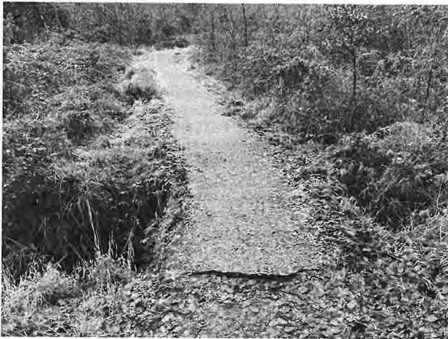
Figure 3. Another section of the existing path showing erosion of concrete.
