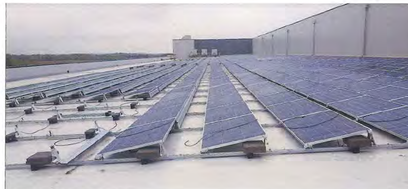
Image of typical PV array (south facing)
