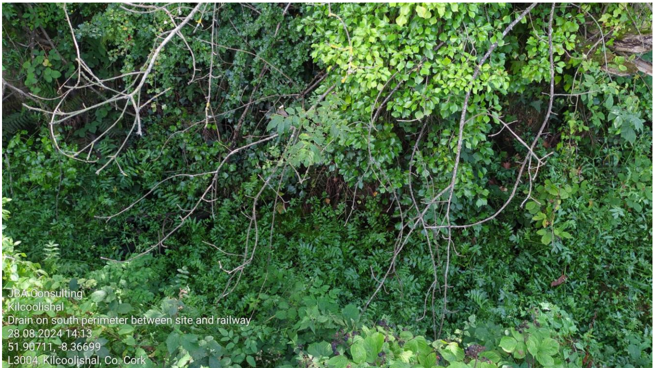
Figure 3-3: Photograph of the overgrown drainage ditch.
